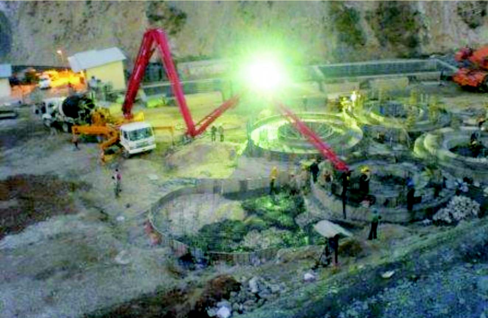
Putzmeister Boom Pump (36 Meter) Of Shakti Commodities working In Alknanda Hydro Electric Project For Construction Of Foundation (Batching Plant Has Capacity 360 Cum Per Hour)
