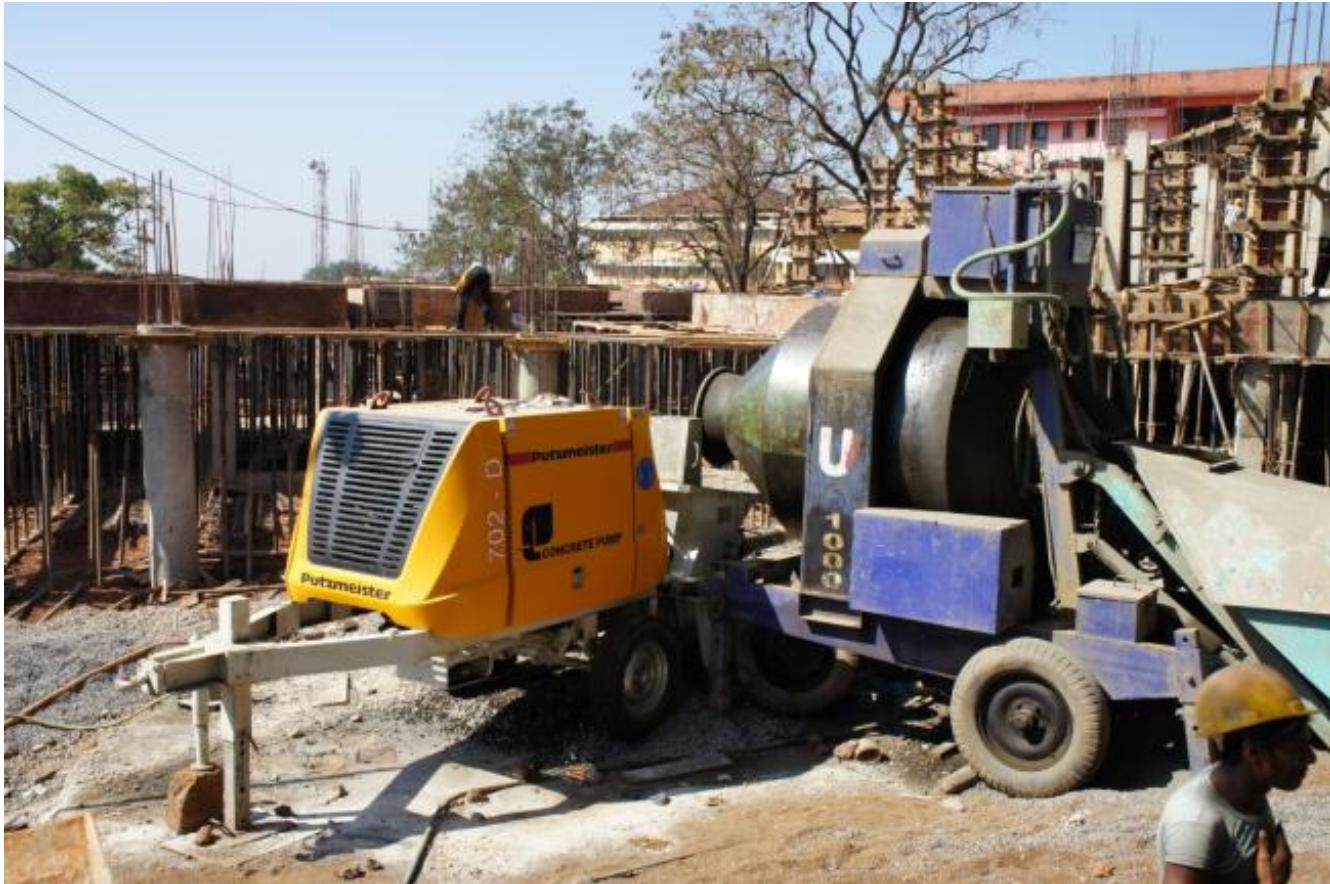
BSA 702D working at the Construction site of Govt. Medical College, Goa
