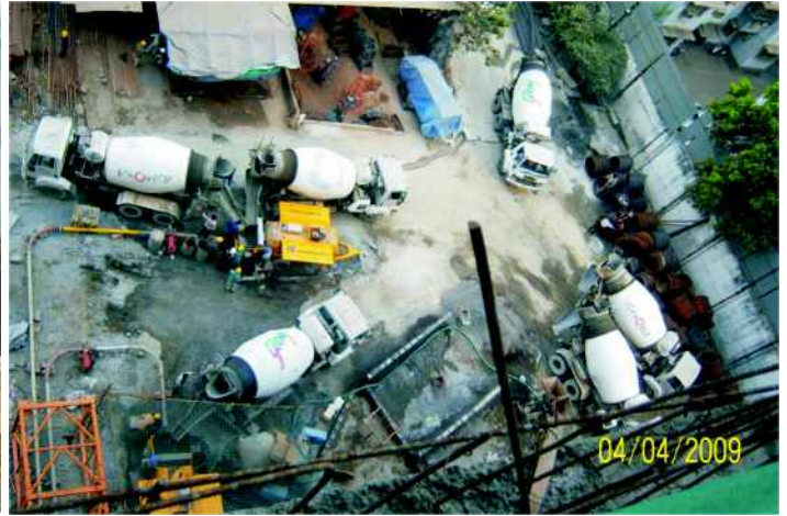
BSA 1408 HD PUMPS SETUP AT SITE
