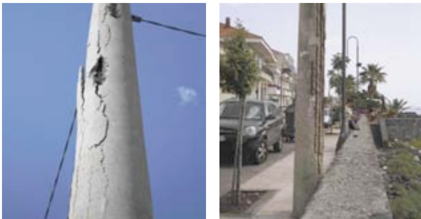
Fig. 17/18: Spalling of the concrete cover due to reinforcement corrosion (severe exposure to sea salt)
