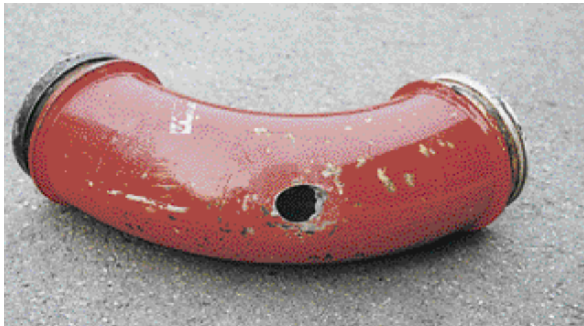
Fig. 31: Pipe wear in the delivery line bend
